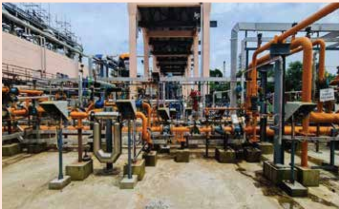
IOCL's new INDMAX fluid catalytic cracking(FCC) unit at its 2.35 million-tpy Bongaigaon
